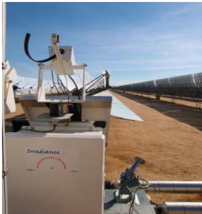
RSR2™ system installed at CSP plant in California
